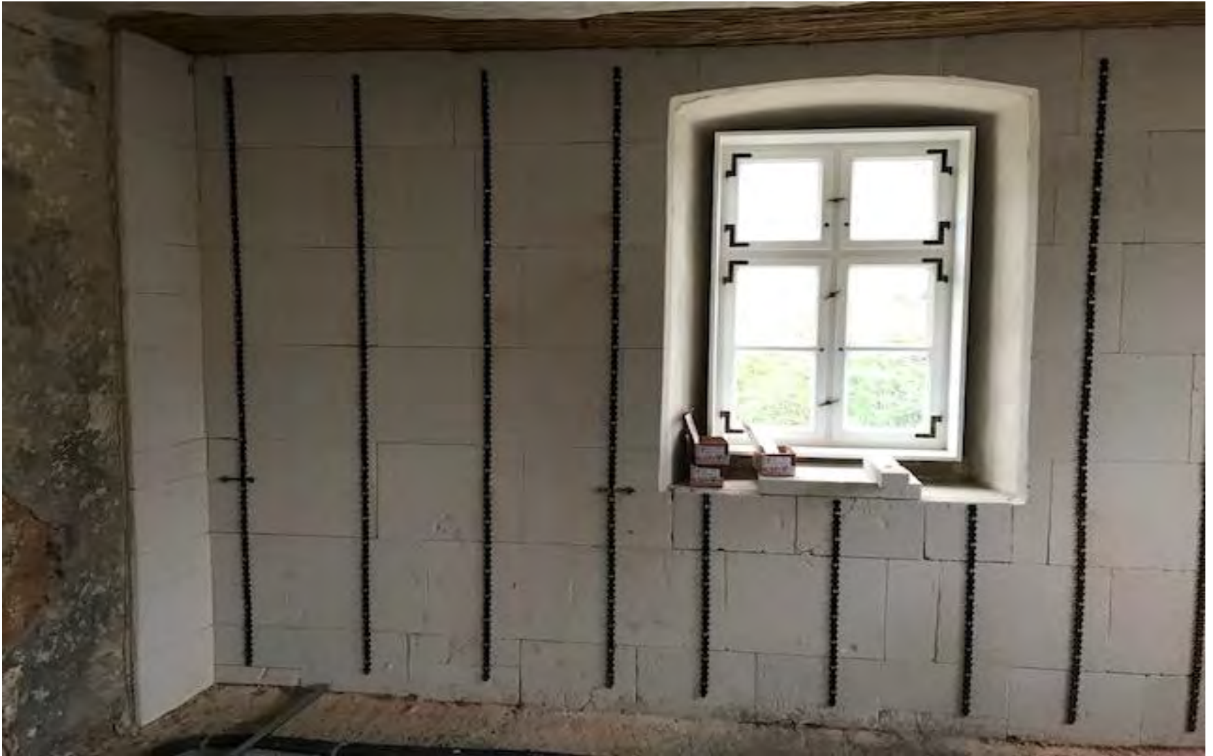
Mineral foam insulation (living rooms) and holders for wall heating pipes
