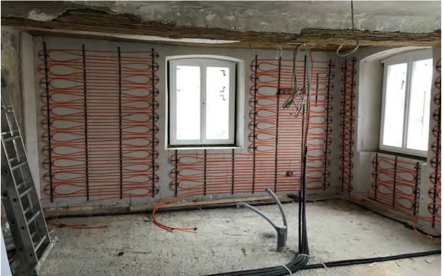
Mineral foam insulation (living rooms) and wall heating pipes
