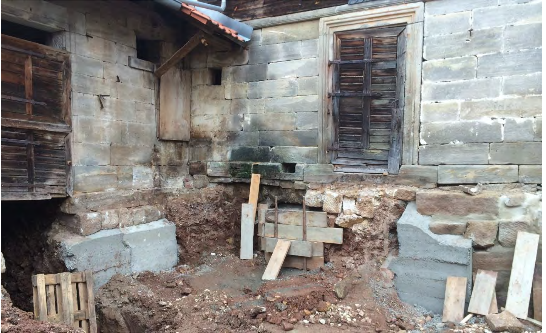
Major damages of the foundation
