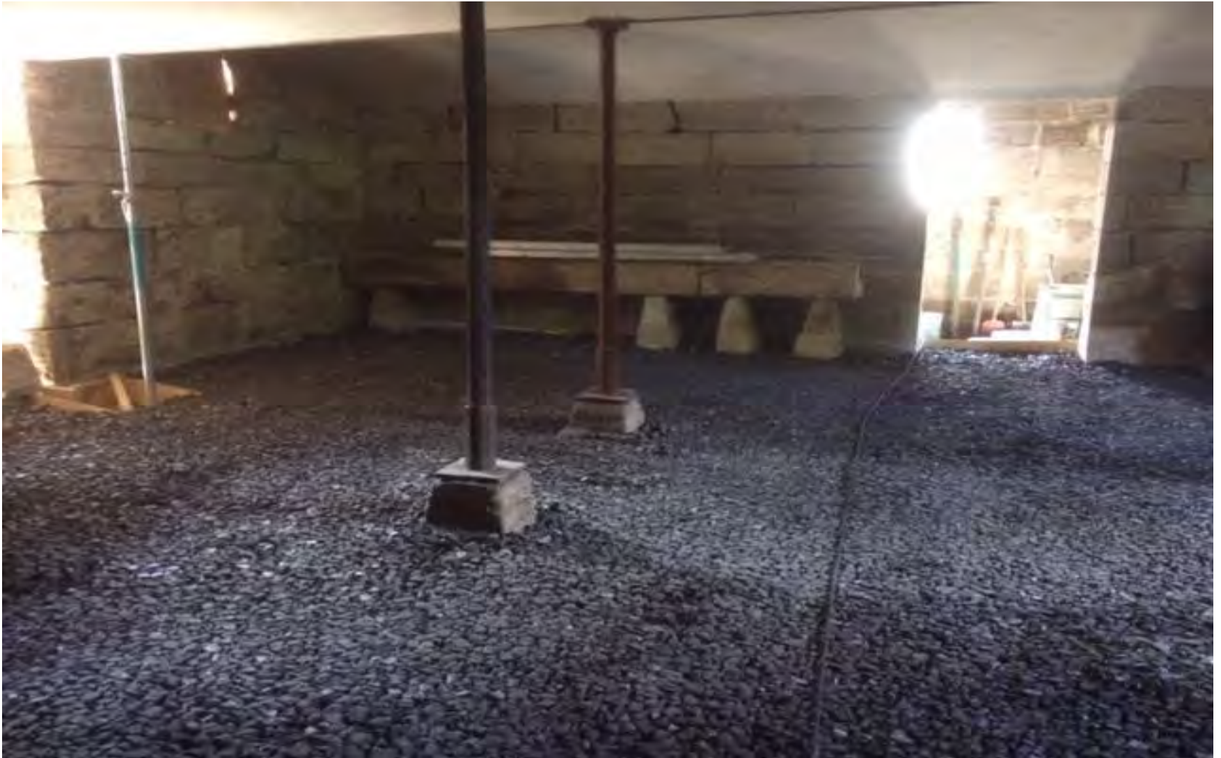
Foam glass insulation (seminar rooms)
