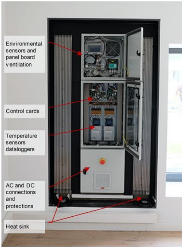
Fig. 9. Front view of the prototype installed in the room. The electric panel is divided into three boards. The bottom one includes the connections, protections and emergency button. The main control and monitoring elements are located in the middle panel. At the top there are external sensor data loggers and the ventilation fan for the board.
